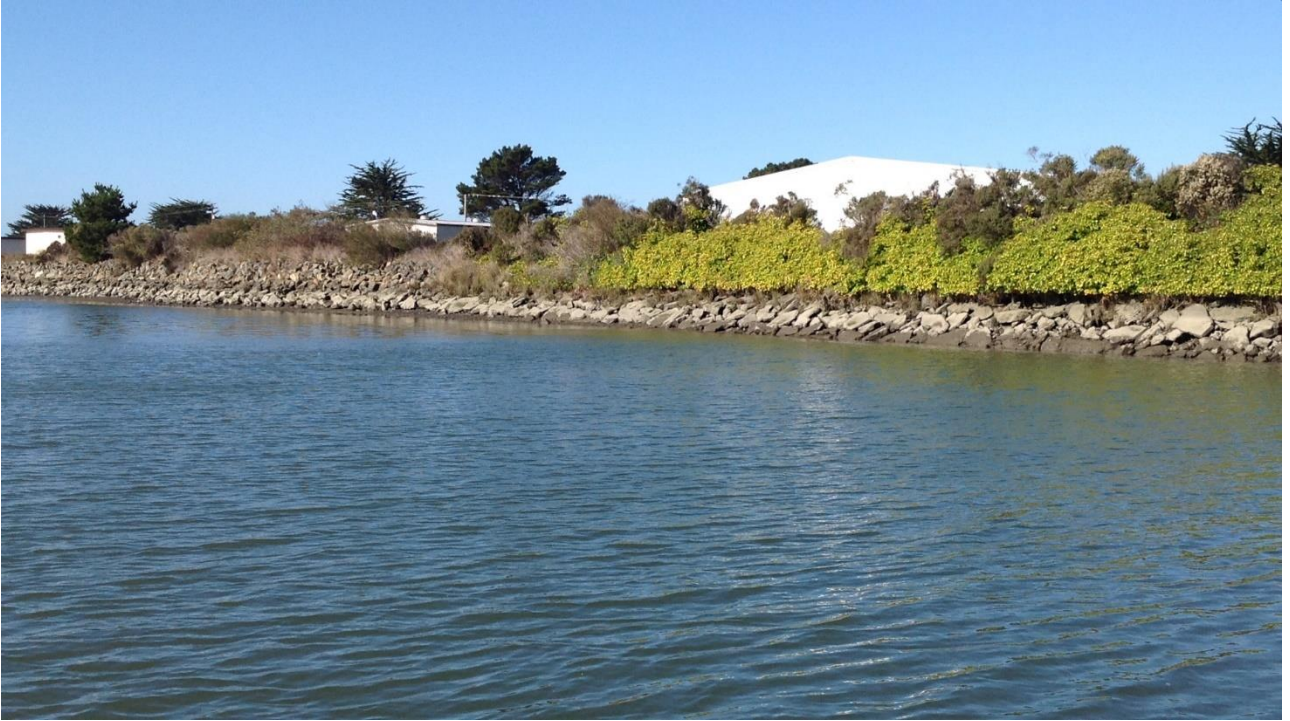
Figure 5. The eastern levee is armored with rock slope protection and concrete rubble.
