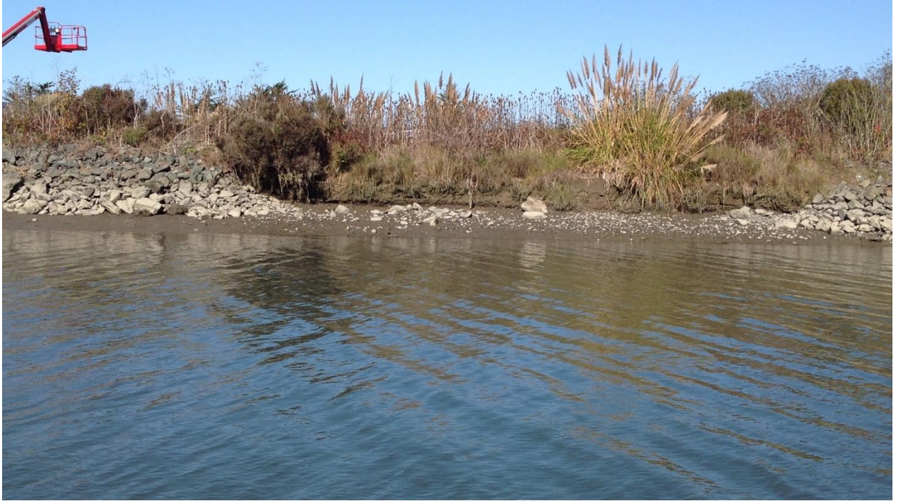
Figure 6. Short Sections of Levee between Armored Sections show Indications of Erosion.
