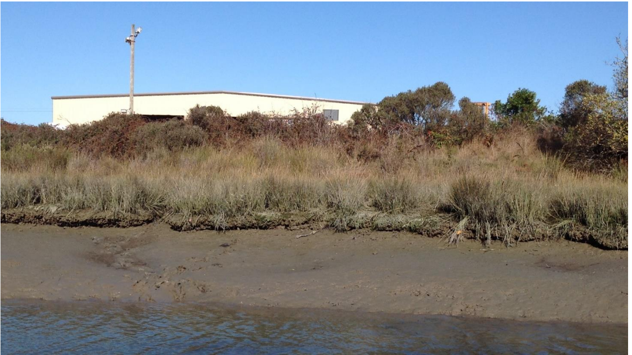
Figure 4. The western levee section is vegetated, fronted by a tidal marsh bench and does not show indications of surface erosion.
