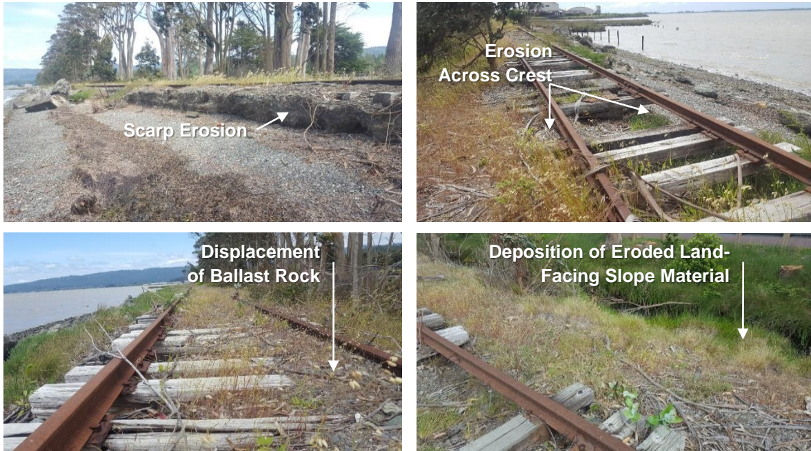
Figure 16. Common indicators of change along the rail prism of the Arcata Bay shoreline.
