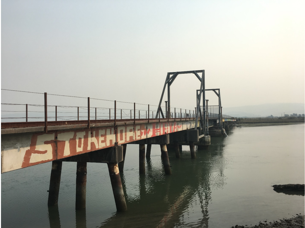
Photograph 6. Trail Segment 2, the proposed trail will utilize the existing railroad bridge over Eureka Slough. Photograph taken October 10, 2017.
