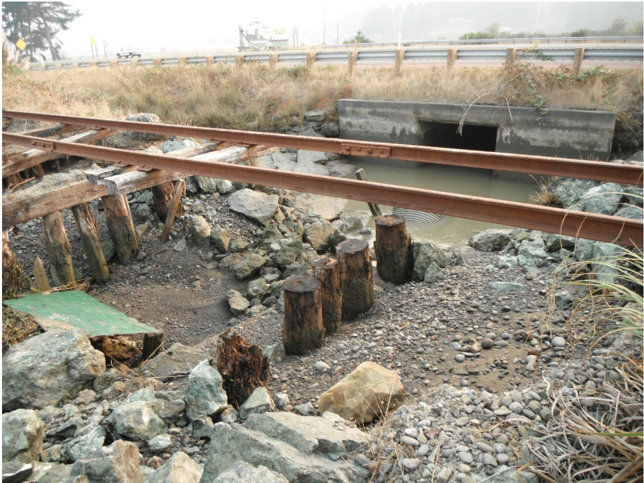
Photograph 1. Current condition of the collapsed railroad grade and culverts at the Brainard's Slough crossing. Photograph taken October 10, 2017.
