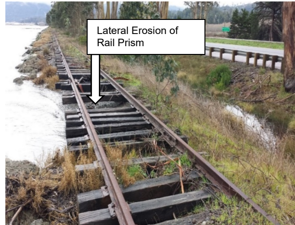
Example Wave-Induced Erosion of Rail Prism Resulting in Displacement of Ballast and Undermined Tracks
