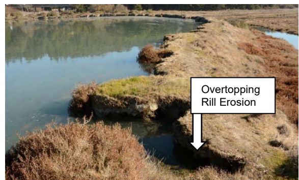
Example Levee Crest Erosion from Repetitive Overtopping (Laird, 2013)
