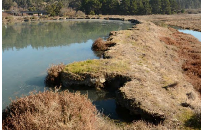
Example Levee Crest Erosion from Overtopping (Laird, 2013)
