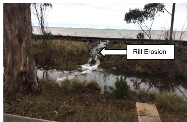
Example Rill Erosion on Rail Prism Top and Backslope Due to Overtopping
