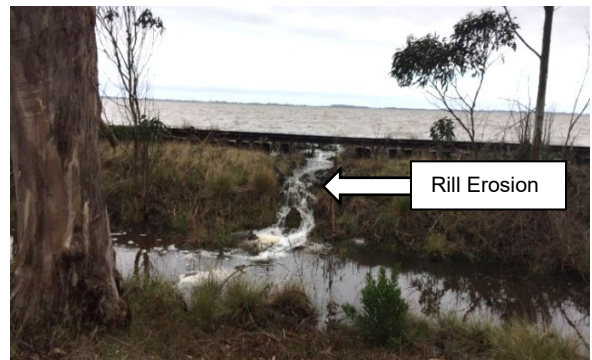
Rill Erosion of Railroad Prism Top and Land-Facing Slope Due to Overtopping
