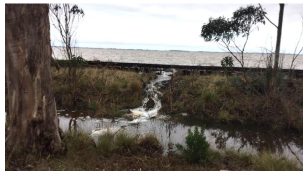
Rill Erosion of Railroad Prism Top and Backslope Due to Overtopping
