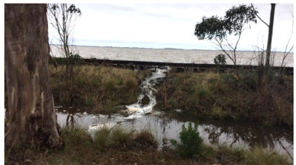
Rill Erosion of Railroad Prism Top and Backslope Due to Overtopping
