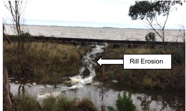
Overtopping Flow at Lowest Point of Rail Prism
