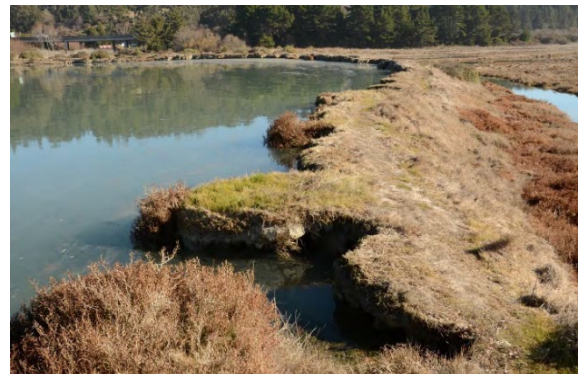
Example Levee Crest Erosion from Overtopping
