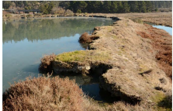
Example Levee Crest Erosion from Overtopping (Laird, 2013)
