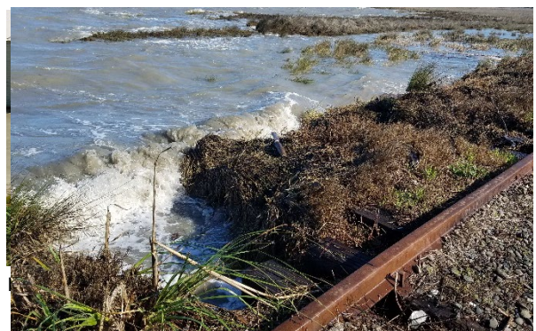
Wave-induced Lateral Erosion along Rail Prism.
