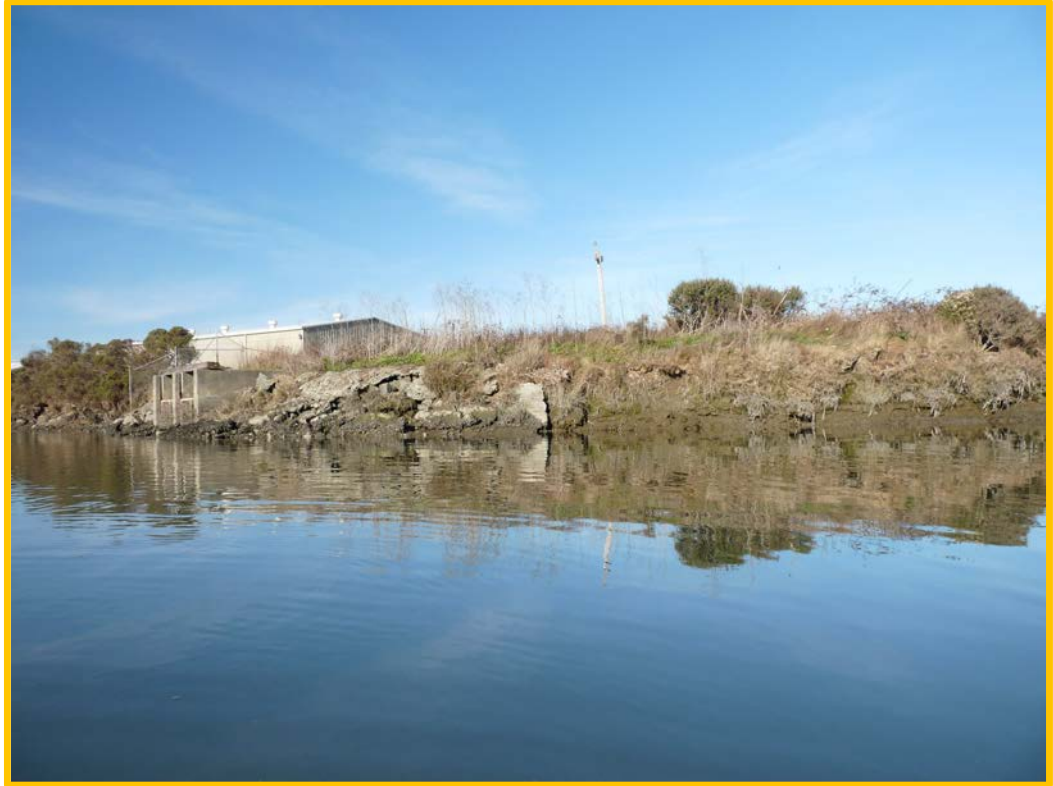
North bank of Eureka Slough with unarmored section on right (Aldaron Laird).
