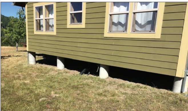
This cabin has good defensible space, though a perimeter foundation would improve the design.
