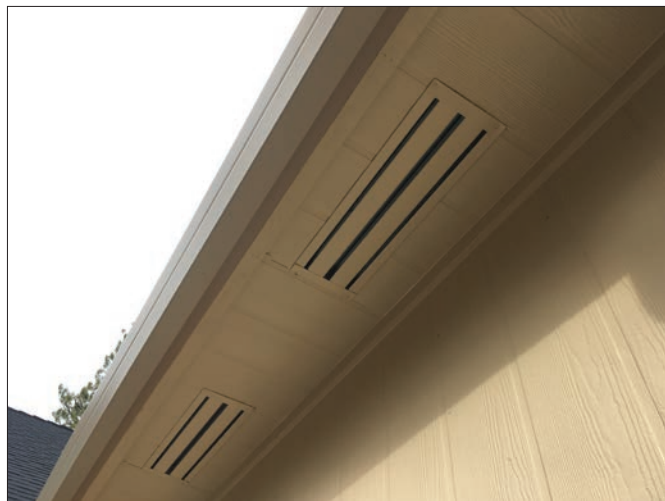
This newly constructed home utilized a soffit eave with a baffle vent that helps resist both flame and ember penetration.
