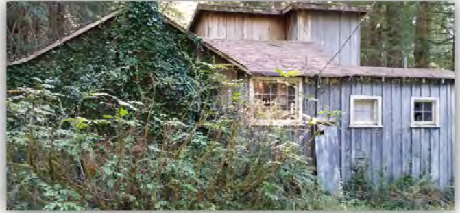
Home with combustible materials and adjacent vegetation, E. Nunez, 2015.
