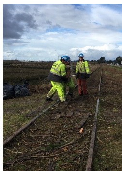
California Conservation Corps members prepare the north end of the Eureka-Arcata Trail for construction.
