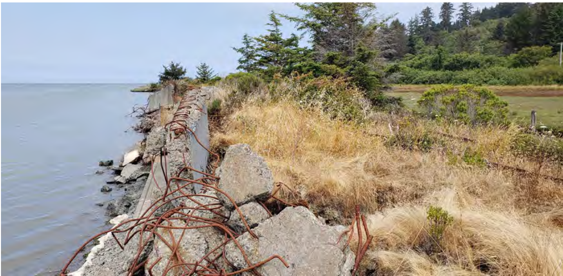
Image 16: Concrete rubble with steel rebar along the shoreline (Segment 3).
