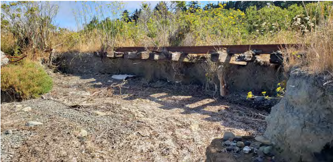
Image 18: Shoreline erosion (Segment 3).
