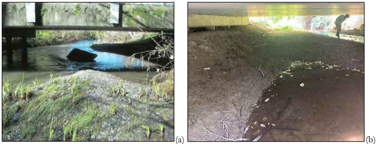
Figure 2-7. Under the northern bay of the Old Arcata Road bridge at Jacoby Creek in (a) March 2006 and (b) September 2021 showing the center bent (left on photos) buried in sediment.
