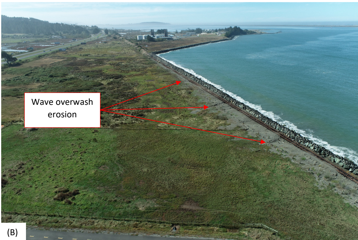
Figure 8. 2022 aerial image of Trail Segment 1 & 2 within a portion of Shoreline Reach 1 (A); and 2023 oblique aerial view of Shoreline Reach 1 existing rock revetment along the proposed Trail Segment 1 (B), note the localized overwash erosion from wave runup and overtopping on the back area of the revetment. Drone image (B) provided by County of Humboldt.
