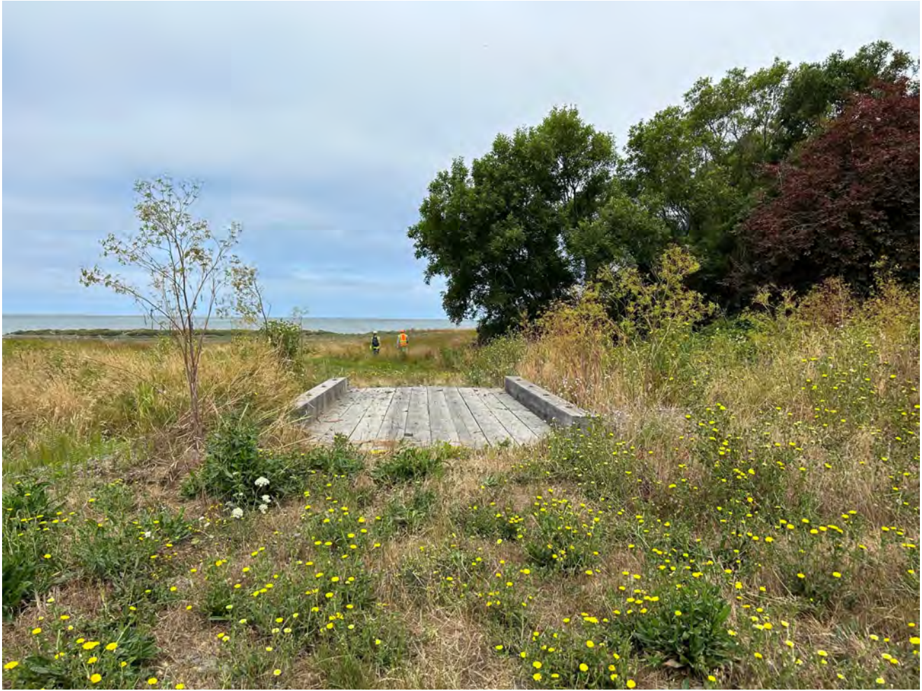
Photo 13. Existing wooden bridge over a tributary of White Slough. Note the wooden bridge is not atop the former railroad alignment.
