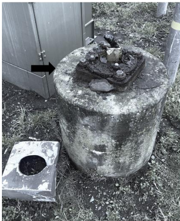
Image 1: Rusted and corroded light pole base.
