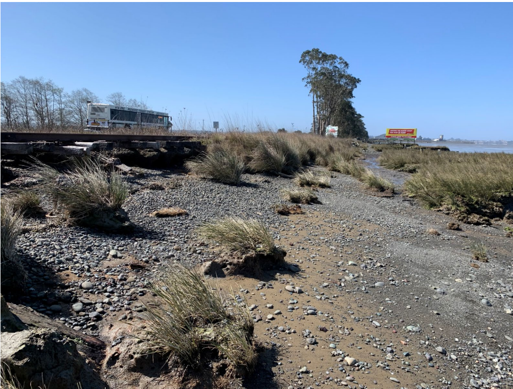
Photo 7. The undercut rail line.
