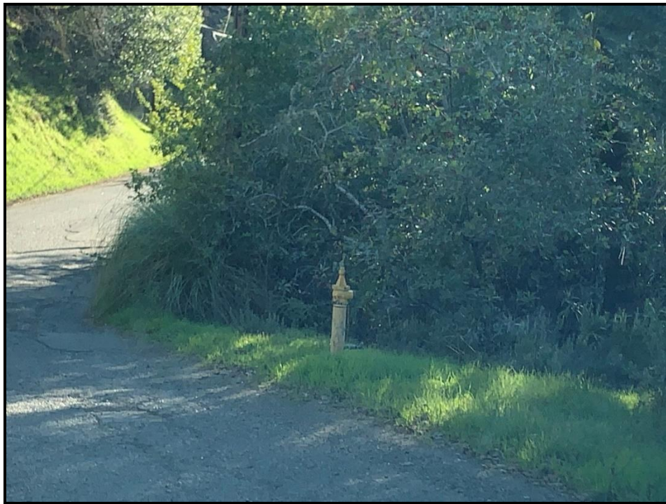
Municipal fire standpipe along Blue Rock Road.
